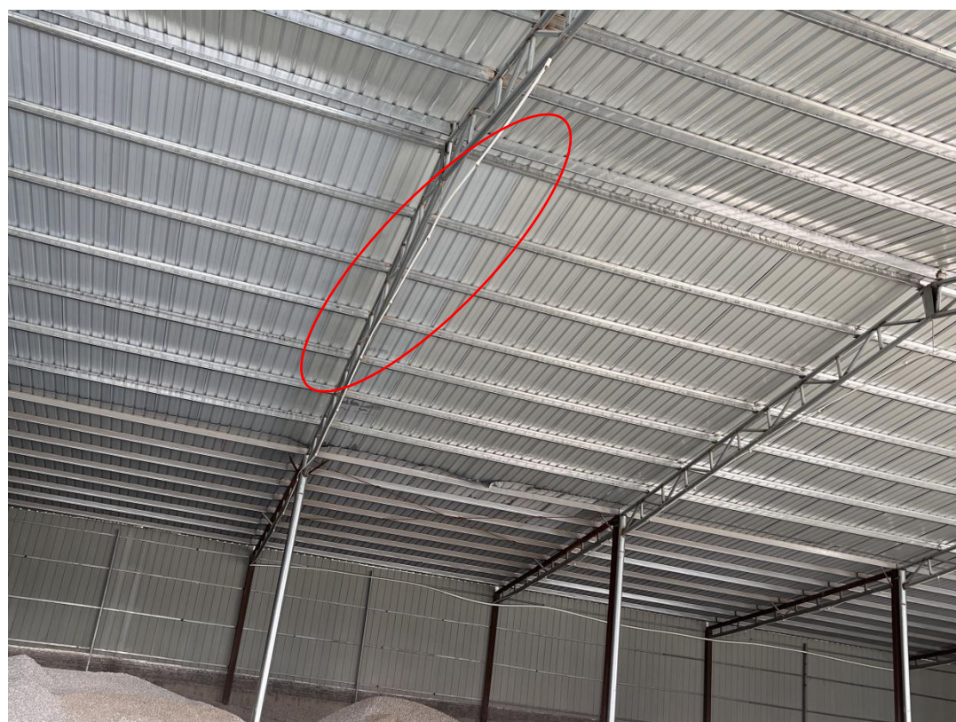
堆场内水雾喷淋
