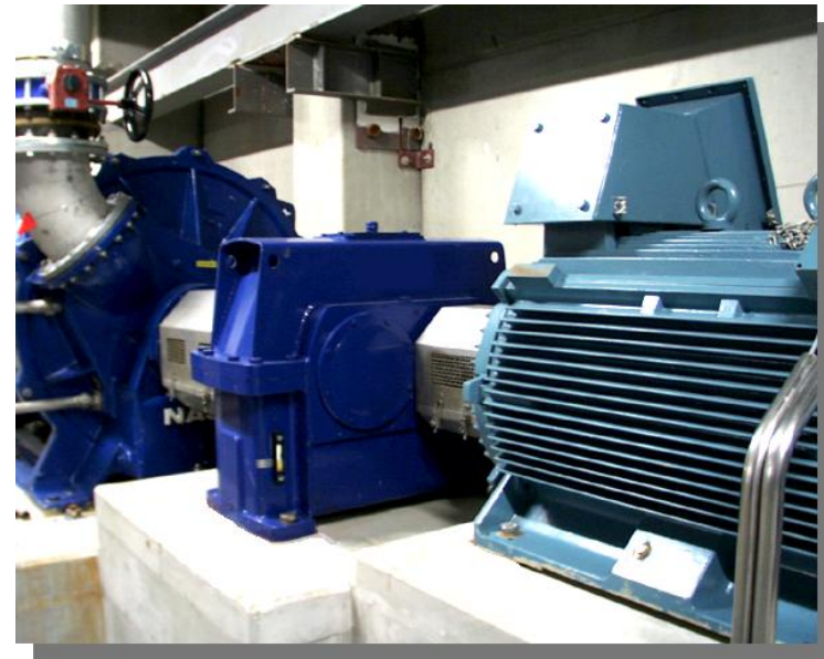
Vacuum pump drive
